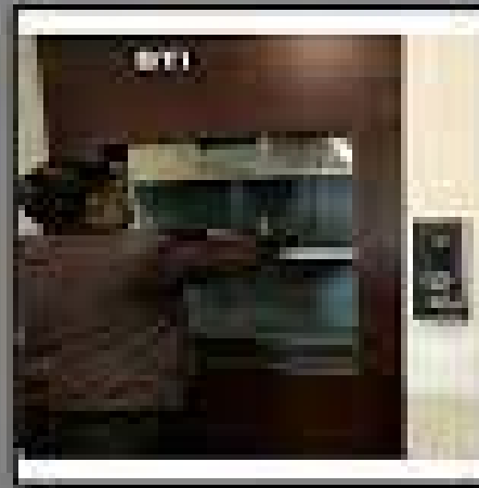
KITCHEN DUMBWAITER LIFT
